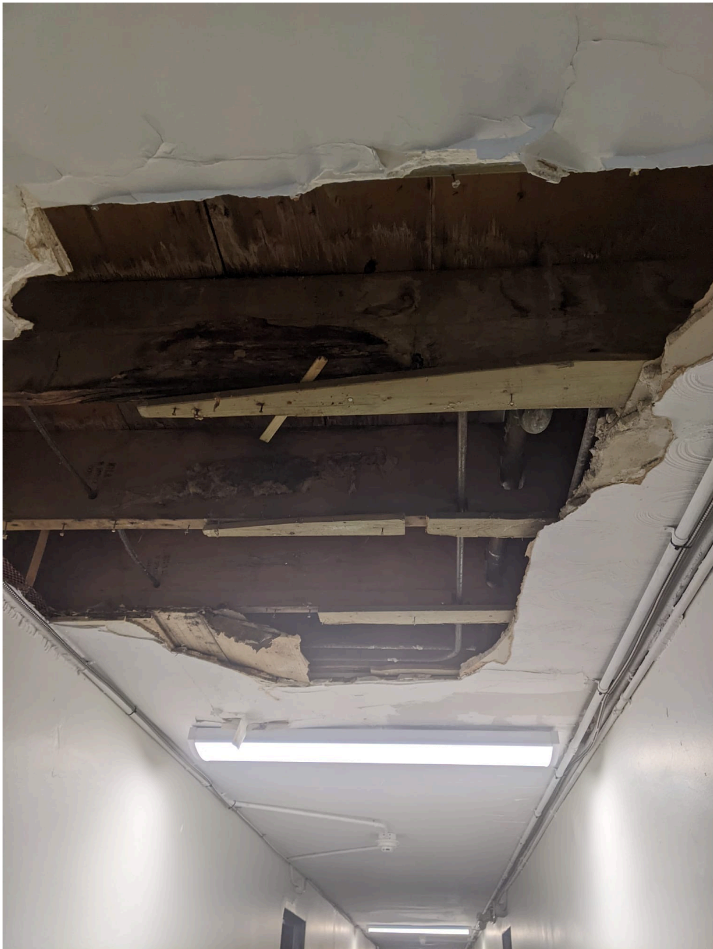
A photo depicts a ceiling that has not been properly repaired and has been exposed over years at Tanya Burkart's townhome complex in Brampton, a result of water leakages that seep into tenants' units.
